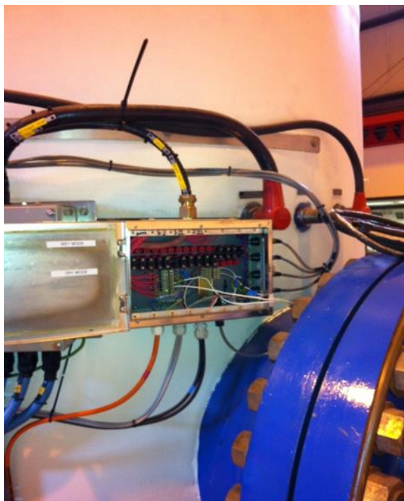
AED External chamber connections for testing
